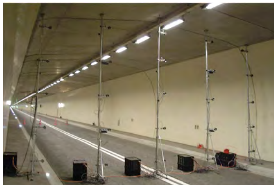
Figure 1. Flow measuring grid in tunnel
