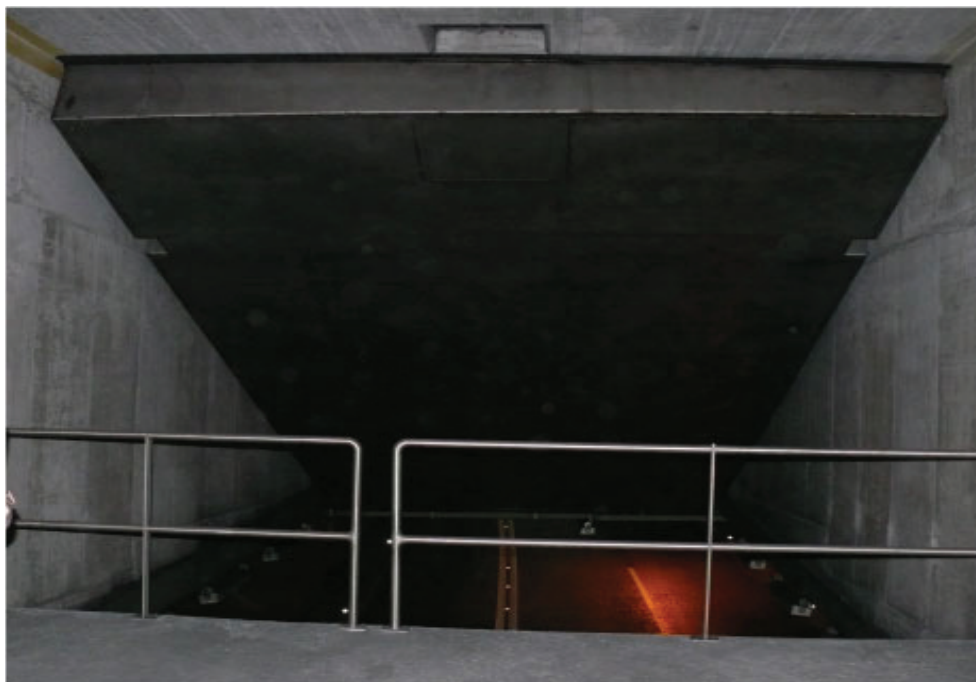
Figure 3.2: Flap gate, used for portal air extraction, open position
